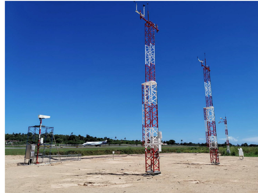
Meteorological Towers – Installed at Samui International Airport by ILLUSTRO
